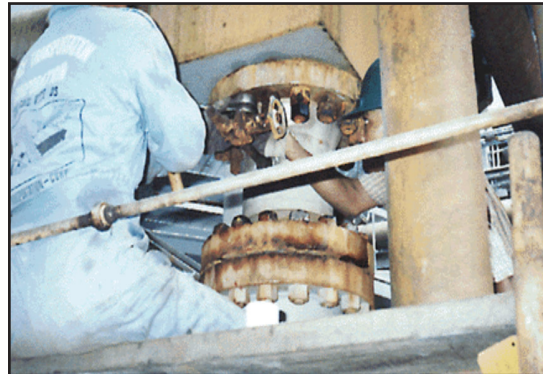
Previously, 3 men with hot work permits were required for 6 hours to disassemble flange bolts.
