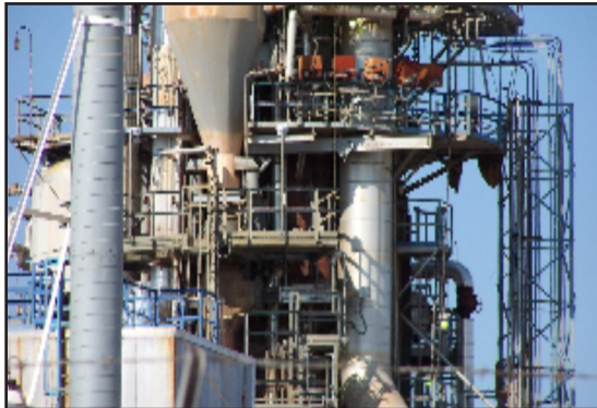
Downtime and loss of production was a critical concern for the customer.
