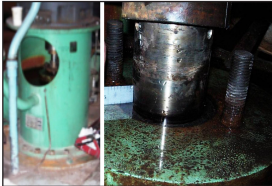
Condensate leaking from the Hotwell Pump had corroded the shaft and pump face.
