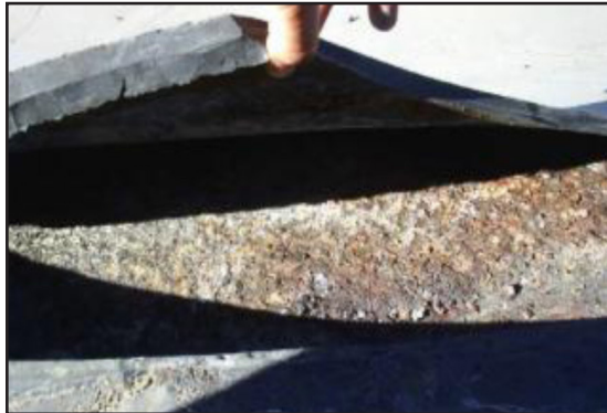
Delaminated rubber liner with corrosion underneath
