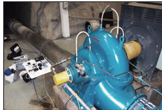
Reinstalled pump undergoing efficiency measurements
