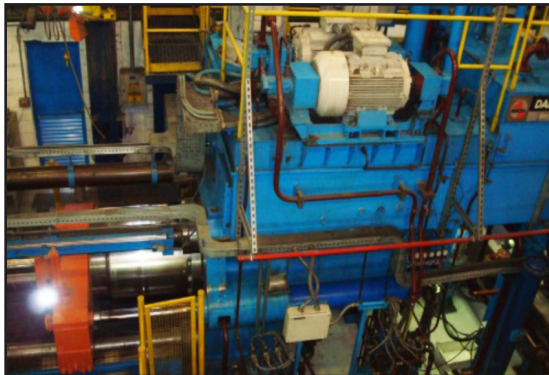
Extrusion Equipment - 950 x 1000 mm (~37 x 40") Pressure - 400 bar (5800 psi) Oil Temperature - 50° C (122 F°)
