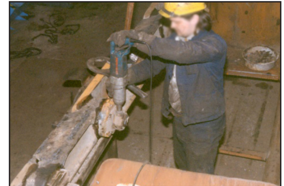
Hinge bolts were easily removed during scheduled maintenance.
