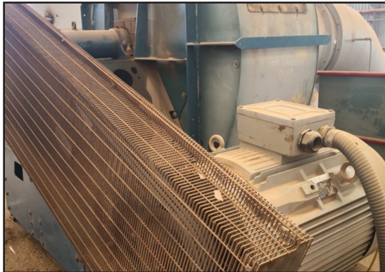
Oven fan motor before service.
