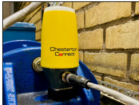
Chesterton Connect sensor unit installed.
