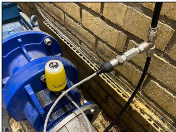
Chesterton Connect set to monitor barrier fluid.
