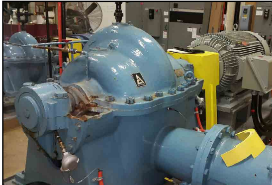
The double seal solution was not effective and posed environmental issues.
