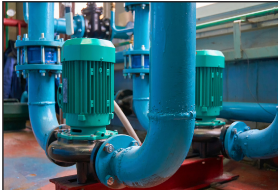
Vertical wastewater pumps.
